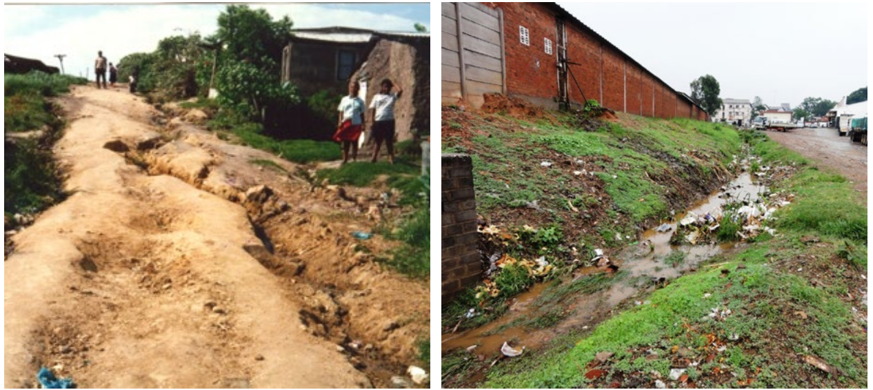
Figure L.9: An example of erosion on an unsurfaced road (L) and lack of maintenance of an open channel (R)
