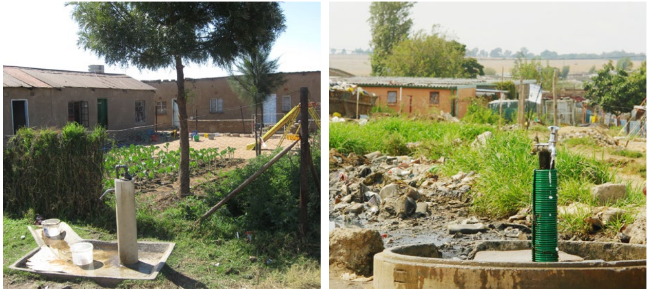
Figure L.3: Excess water at a communal standpipe redirected for garden use (L) and excess water causing erosion (R)
