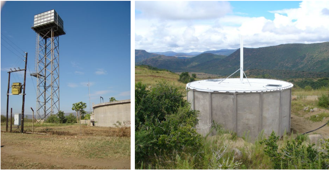
Figure J.3: Examples of concrete and metal reservoirs (L) and a concrete reservoir (R)
