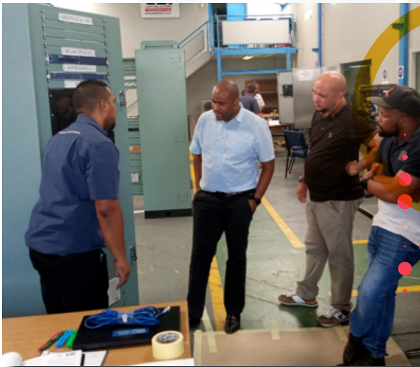
Factory Acceptance Testing of Human Machine Interface panels, March 2023. In the centre, Mr Duma Mhaule, Director: Electrical Engineering Services, and the KDM Project Manager, Mr Brendan Pillay on left, with staff from Control SI, illustrating the built components.
