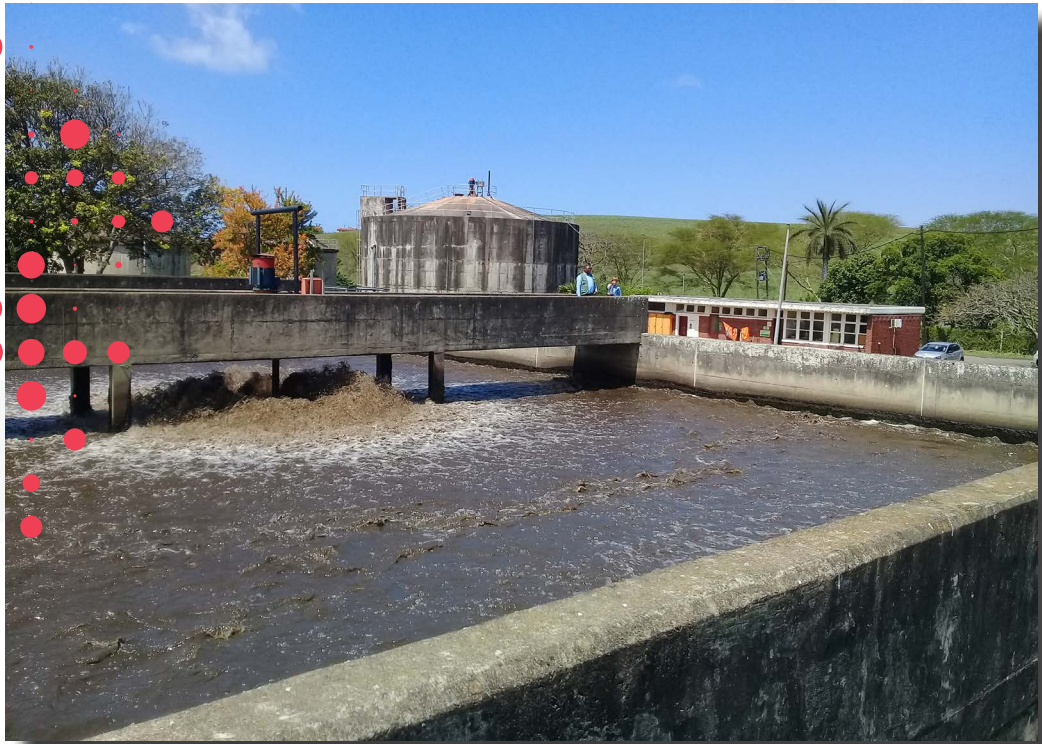
The Sundumbili Water Treatment Works
