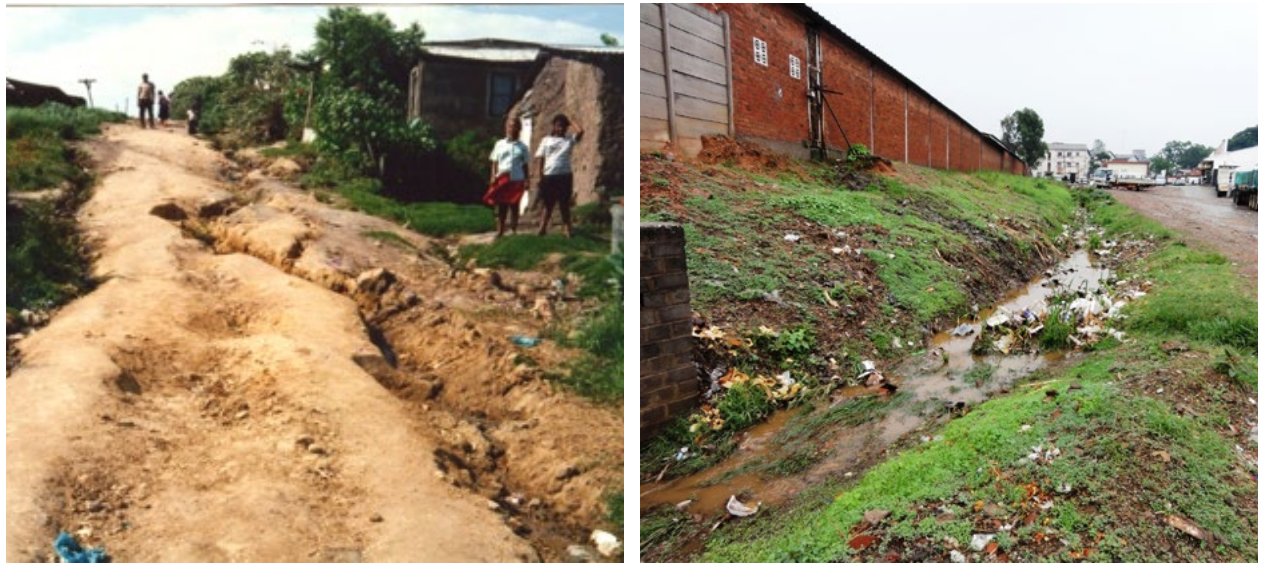
Figure L.9: An example of erosion on an unsurfaced road (L) and lack of maintenance of an open channel (R)
