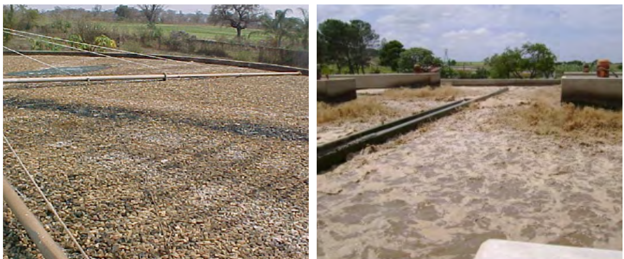
Figure K.3: Biofiltration treatment plant (L) and activated-sludge treatment plant (R)
