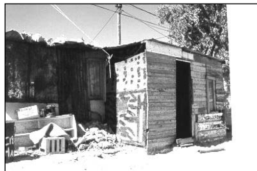
Photo 6-16: Poor structural condition
