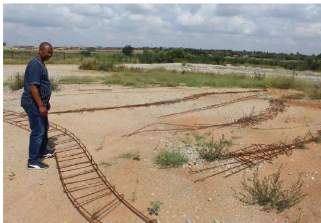
Photo 3.2. Unused building material left to rot over a year –R6million been wasted on unfinished project to construct an EMPD precinct in Boksburg
