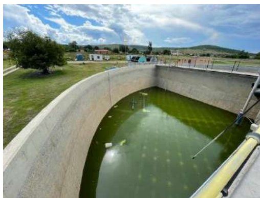
Photo 6.6. Sewage plant in Swartruggens, built in 2012, which is in a state of disrepair.
