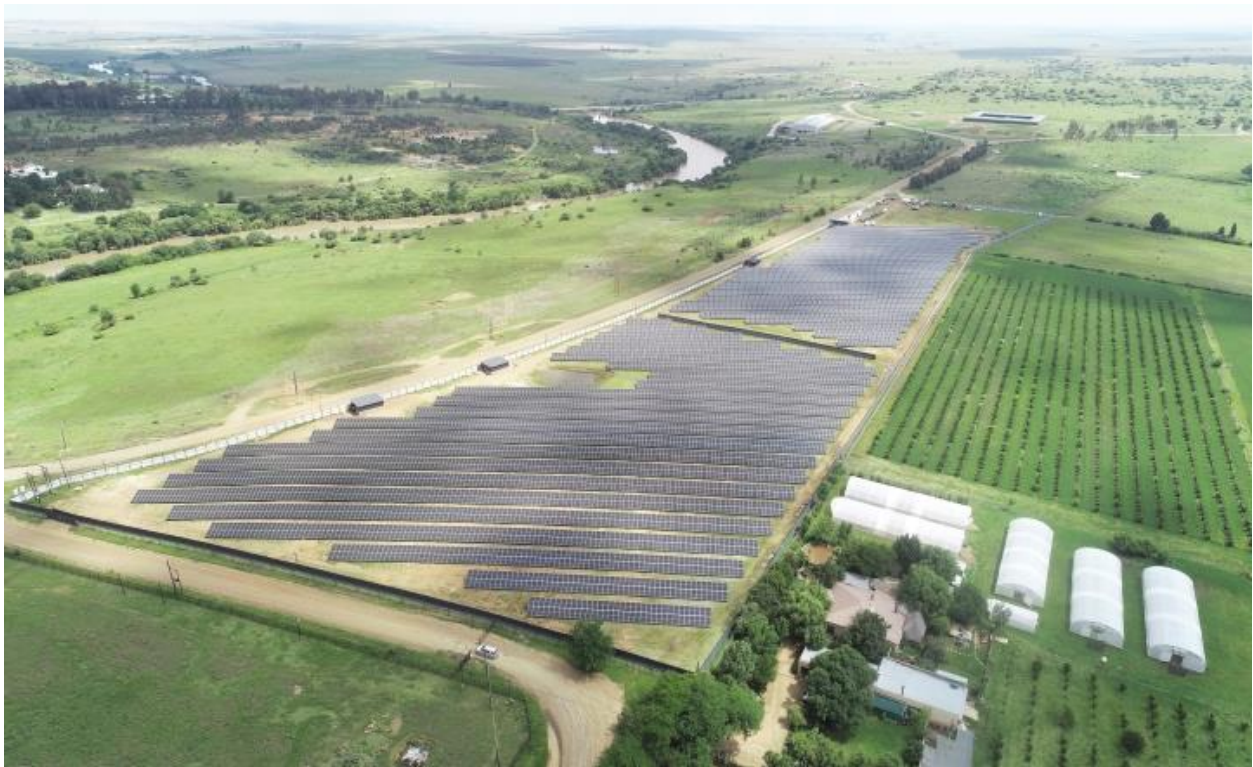
Solar panels installed at Tweeling by Rural Free State on January 20, 2023 in Frankfort, South Africa. It is reported that the private company has been managing the Mafube municipality's electricity network extremely successfully since 2011, the company has replaced substations, built solar farms and also replaced power poles. (Photo by Gallo Images/Rapport/Elizabeth Sejake)
