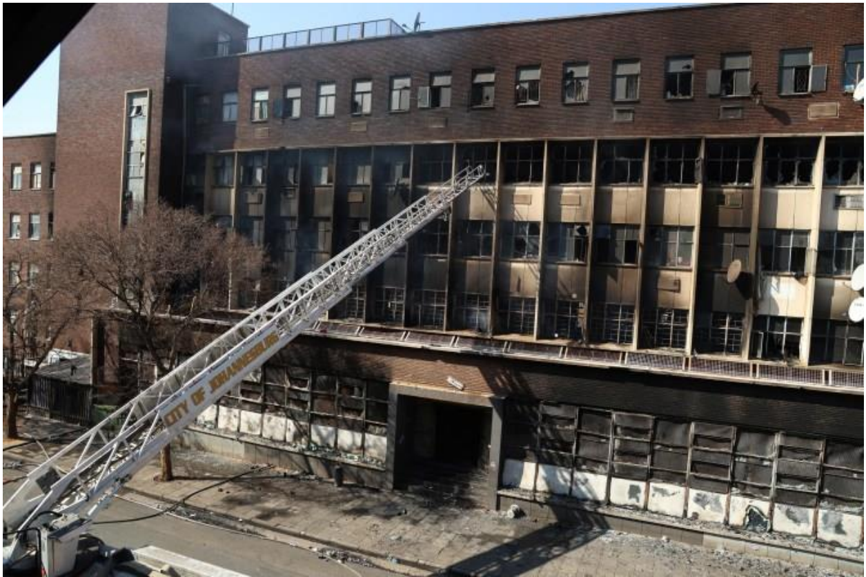
The smouldering five-storey Johannesburg CBD building on the corner of Alberts and Delvers streets. (Photo: Felix Dlangamandla)
