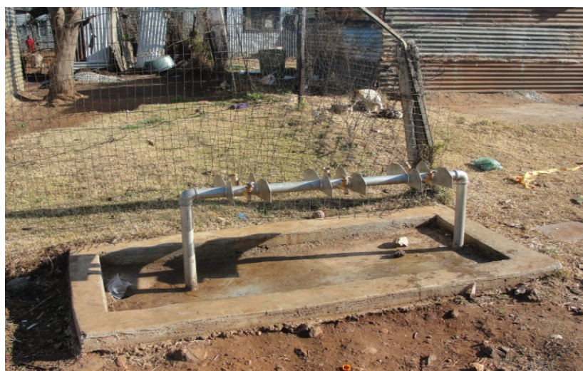
Figure 4: The multiple standpipes with a soak-away area installed by the City in regularised settlements
